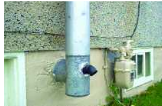
Water heater vent installed through a 'B' vent
