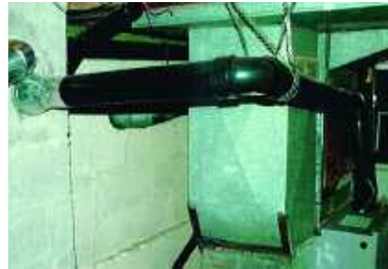
Mid-efficiency furnace vented into masonry chimney
